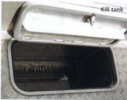
CO 2 fire suppression system
